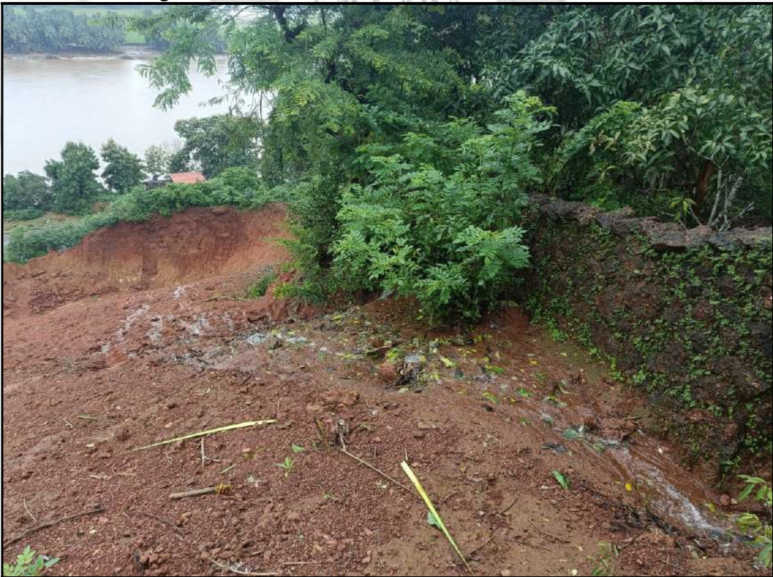
Fig. 1.16: Unguided surface water flowing along the slope above the Ch. no. 147.500
