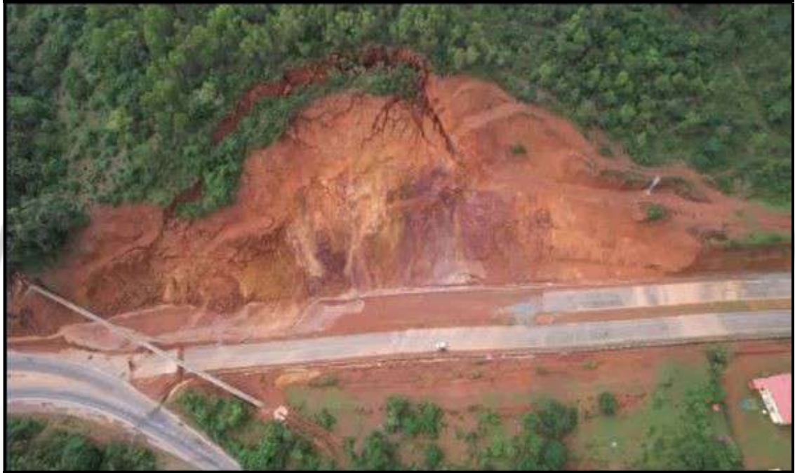
Fig. 2.7: Drone footage showing the recent landslide scar at 166.250
