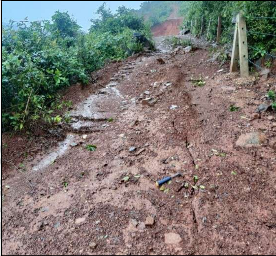
Fig. 1.11: Tension cracks at lower elevation of the left flank of the slide
