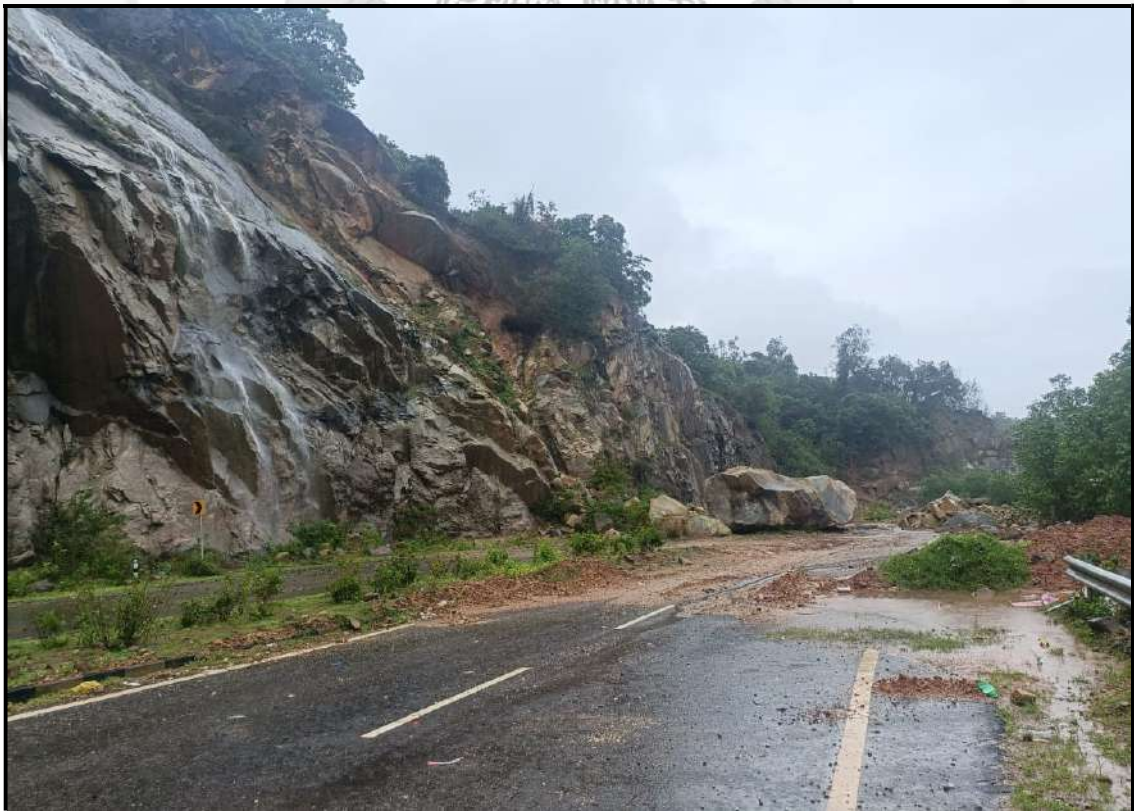
Fig. 2.3: Rockfall incidence at chainage 111.400
