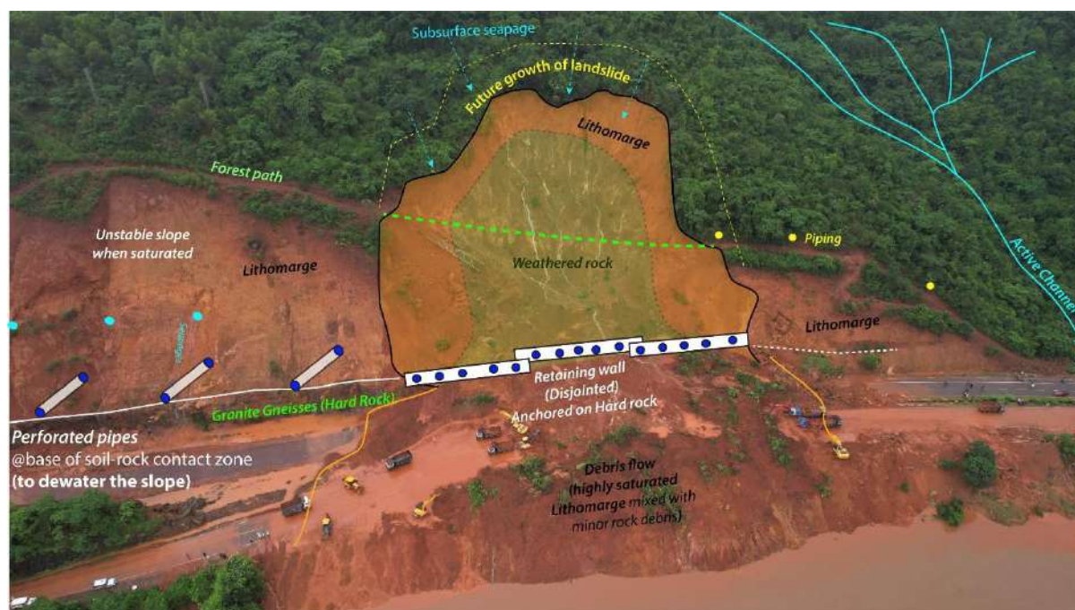
Figure 9: A schematic diagram of the landslide zone stabilization strategy. The Disjointed Retaining wall, anchored to the hard rock , should have provisions for dewatering and extra protection by putting a two-layered configuration in the middle of the landslide zone . Perforated pipes are among the most commonly employed dewatering strategies for reducing the oversaturation in the soil.
