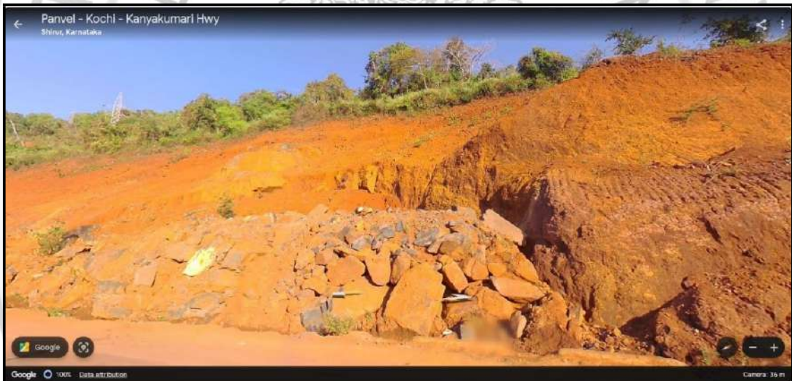
Fig. 1.9: Slump as seen through Google Street View of the Shirur landslide site
