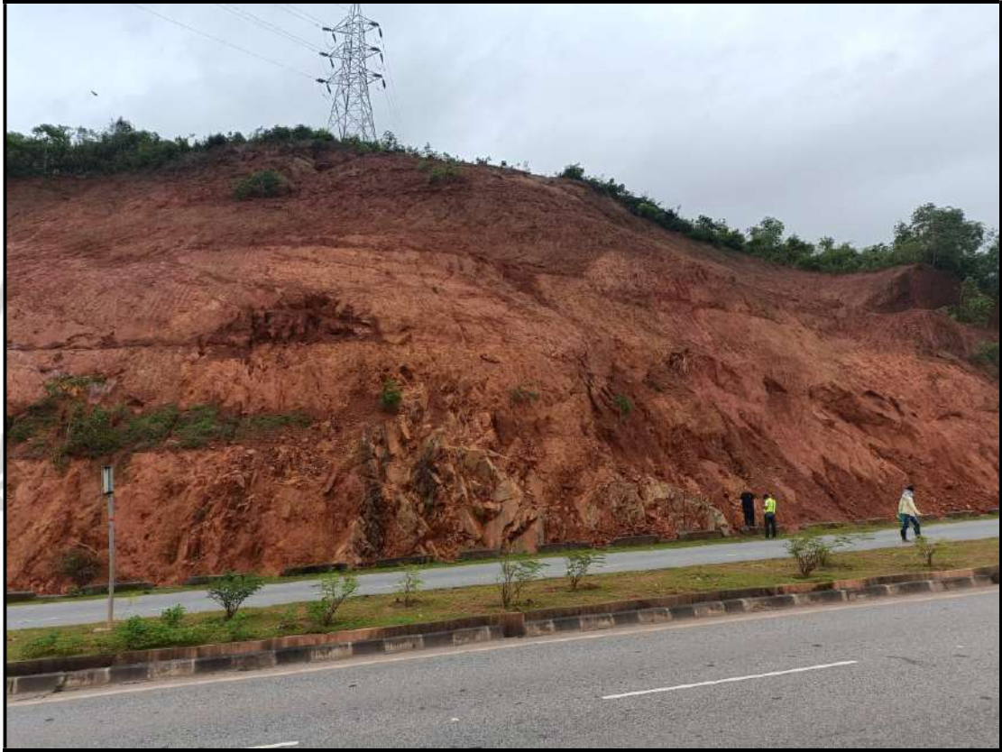
Fig. 2.9: Slope cut at chainage 168.700 showing the debris and minor scars
