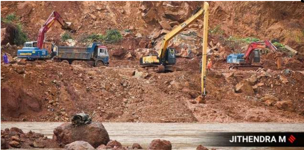
The landslide site on NH-66 in Ankola. (Express photos by Jithendra M)
