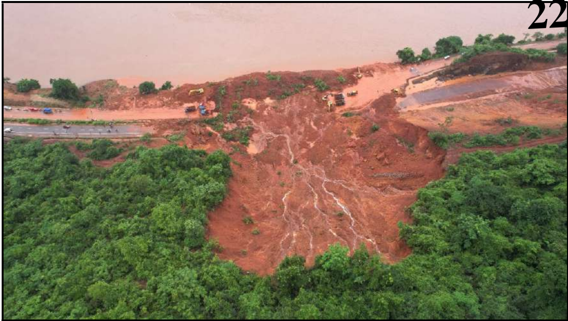
Fig. 1.2: Aerial view of Shirur landslide blocking the communication corridor NH-66 (courtesy IRB)
