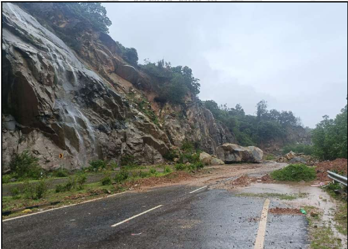
Fig. 2.3: Rockfall incidence at chainage 111.400
