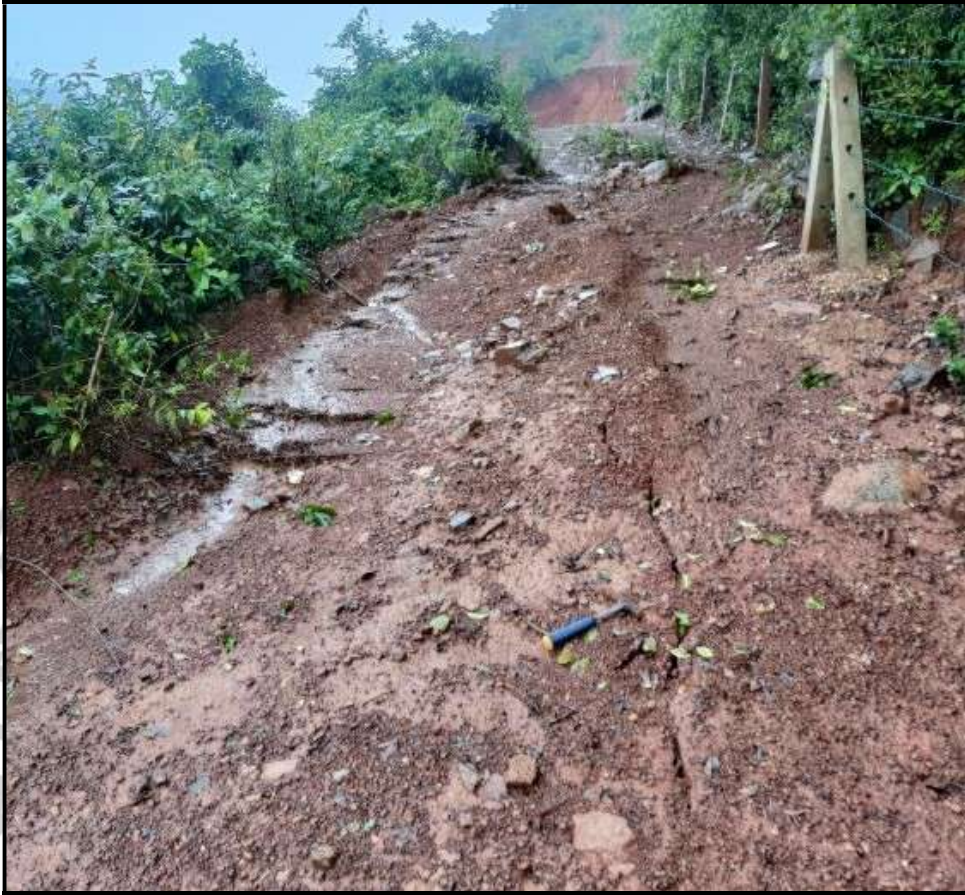
Fig. 1.11: Tension cracks at lower elevation of the left flank of the slide
