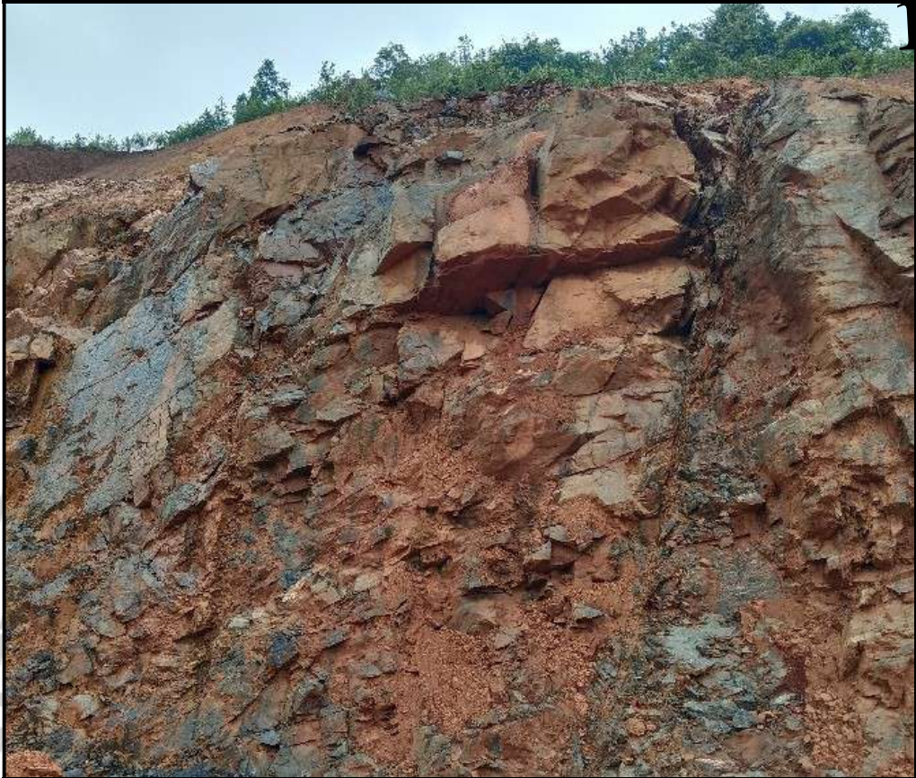
Fig. 1.3: Pyroxenite exposed at the base of cut slope section near Shirur landslide
